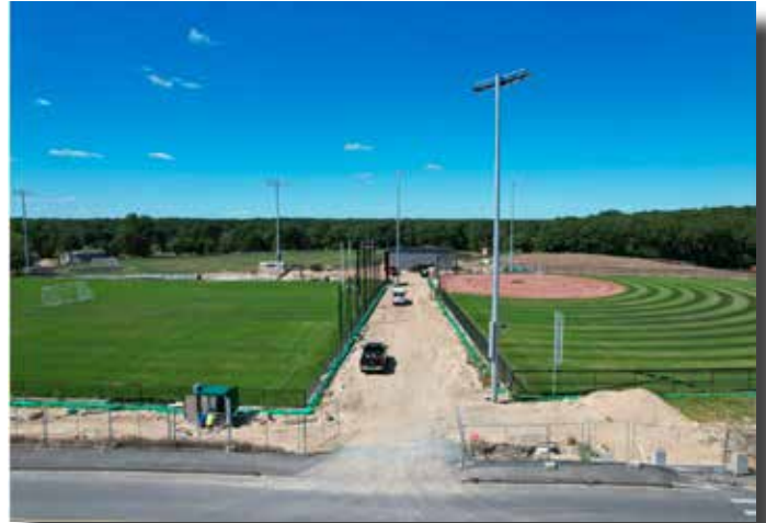
Two new athletic fields are in progress as additions to the existing sports complex.
